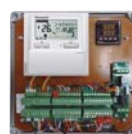
PCB, Power trans, Terminal block
